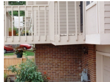
Cantilevered decks have no support columns to ground
