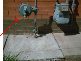
Pressure valve to left of meter may burp a small amount of gas
