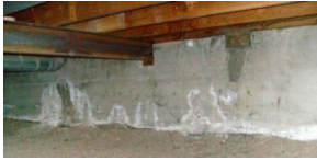
Spalling on inside of crawlspace wall
