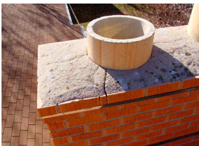
Cracked cap and no spark arrestor
