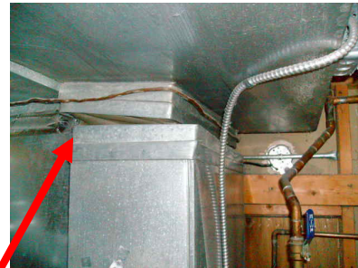
Expansive soil causes movement seen at furnace
