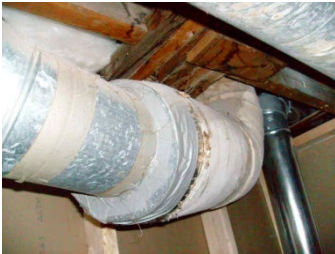
The tape on the joints may contain asbestos the insulated wrap almost certainly does
