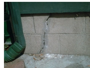
Downspout problems can become foundation problems
