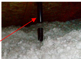
Sewer vent pipe not connected
