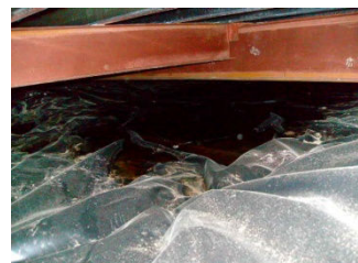
Water leaking into crawlspace from toilet above
