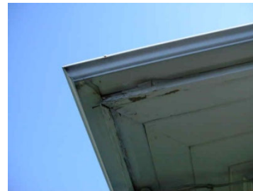
Leaking gutters can rot fascia and soffit
