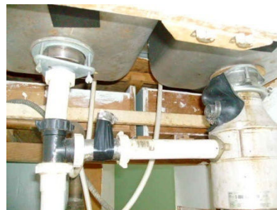
Sink drains should use plumbing parts only
