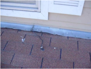
Damage from water and snow driven under flashing
