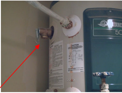
No extension on pressure release valve
