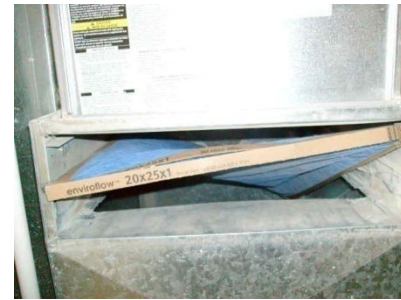
Improper filter installation
