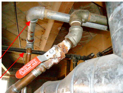
Copper to galvanized iron pipe connections cause corrosion
