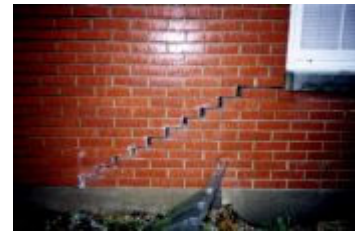
Bad drainage can cause bad cracks
