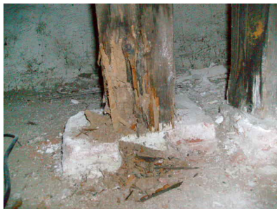
Rotted support post
