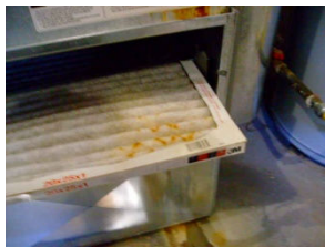
Condensation dripping onto filter grows mold
