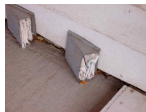
Blocked crawlspace vent
