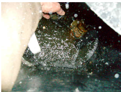
Sump full – pump not working
