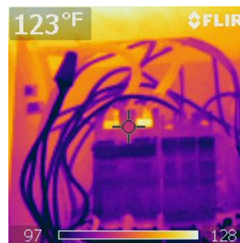
Handyman electric work Infrared shows it's hot enough to catch fire - 128° F
