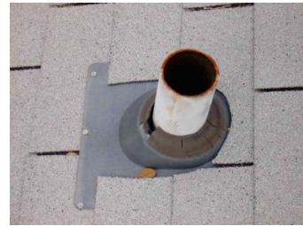
Worn out rubber flashing
