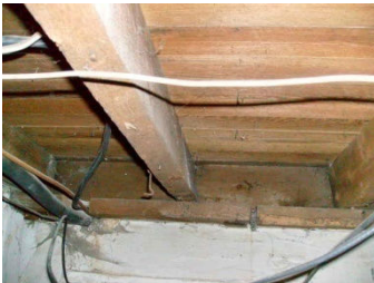
Twisted floor joists
