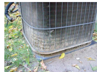
Keep condenser cooling fins clean with a garden hose
