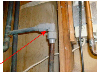
Polybutylene plumbing connection – known to fail
