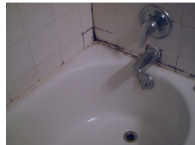
Sometimes caulk needs replacing
