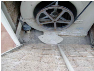
Inside a swamp cooler
